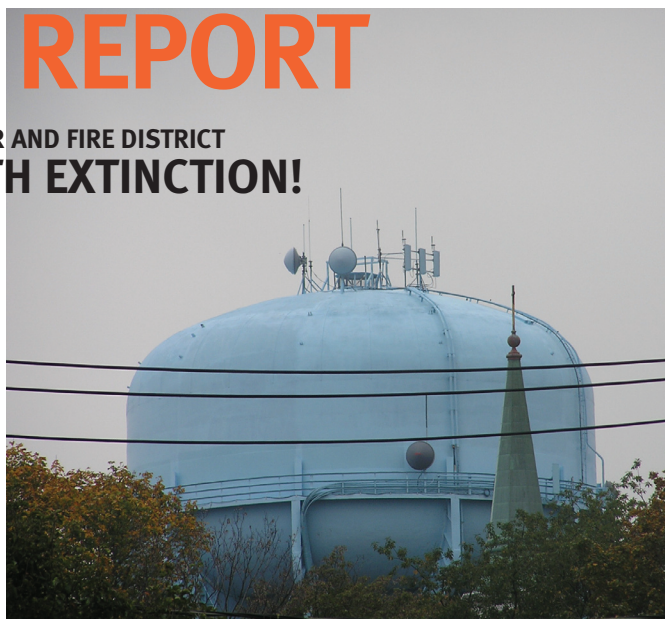
Existing Nassau County radio equipment atop the Thomaston tank.
