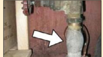
Lead service lines are usually connected to residential plumbing using solder.
